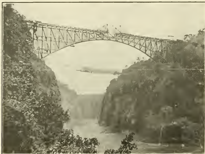
VIEW OF ZAMBESI GORGE AND BRIDGE JUST AFTER LINKING TOGETHER OF THE TWO HALVES.
